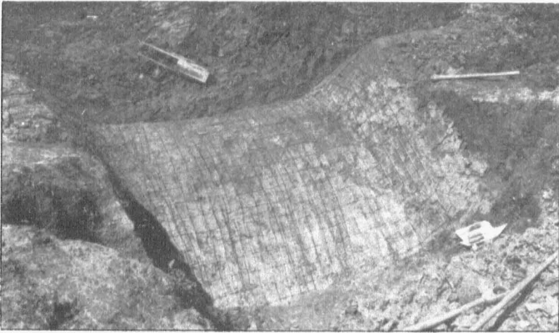
Fig. 2.—Downstream side of shaped earth form. This earth form at the end of a terrace outlet is ready to be covered with concrete and will carry water from a terraced field in Scotland County. Notice the heavy hog wire which will be in the middle of the 4-inch layer of concrete.
