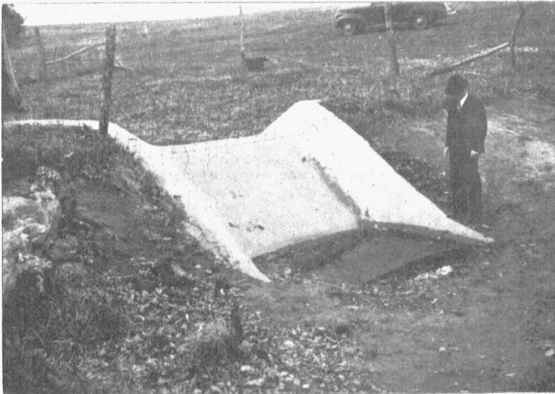
Fig. 10.—This Missouri dam carries water from approximately 30 acres of terraced land. The water comes to it through a broad constructed grassed outlet 34 feet wide along the field boundary to the left. Notice the water standing in the stilling basin below. The velocity check which is here submerged has prevented the discharge flow from scouring out the channel of the main drain below.
