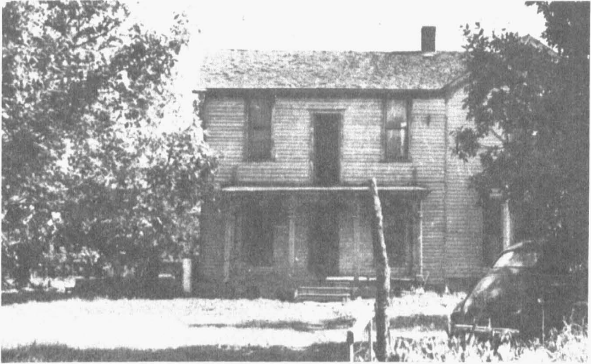
Fig. 4.—Need of repairs and paint oftentimes marred the appearance of old houses that were fairly adequate in other respects.
