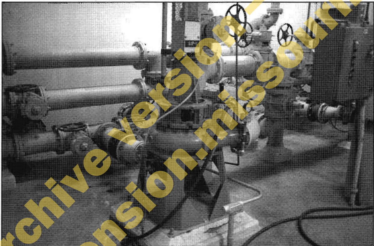
Figure 1. Large electric pumps are used to transfer biosolids to the field in on-site operations.
