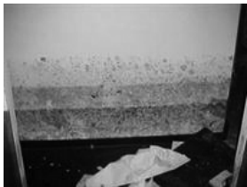
Mold on wall extends above flood level because the moisture wicked up the drywall.
