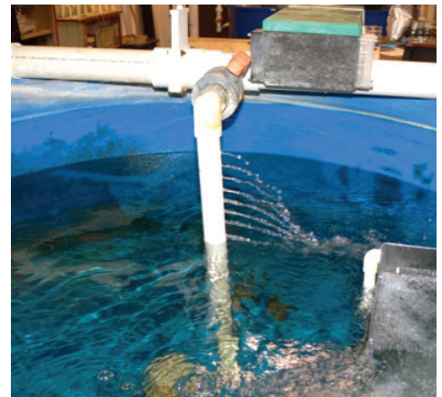
Figure 8. A valve (orange-colored) leads to the water inlet pipe that is submerged in each tank.
