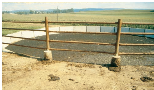
Figure 4. Floating bedding covers the surface of this concrete manure storage tank. The fence prevents accidental entry.
