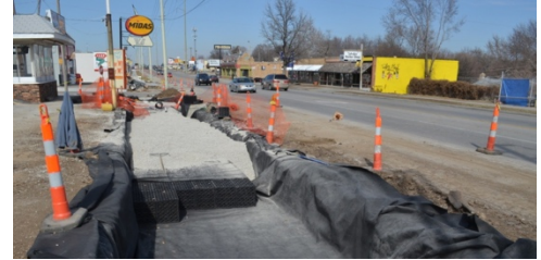
Figure 62 Photo of Bioretention Cell with Below Grade Storage on Troost Street (Source: Dods, 2012)
