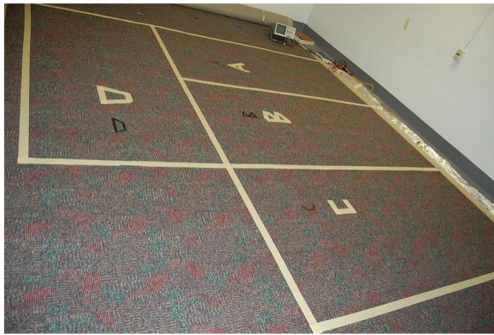
Figure 3.7: Top carpet layer of the sensor layout. The carpet is marked according to the installation segments laid underneath it. Segments A, B, C and D indicate the four installation segments from which the wires are drawn to a common location.
