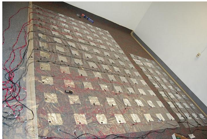
Figure 3.6: Figure above is the sensor layer of the installed floor. The layout consists of 128 sensors placed in group of four installation segments consisting of 32 sensors arranged in 4x8 matrix formats. All the wires from the sensors are drawn to one location where the electronics unit was installed.
