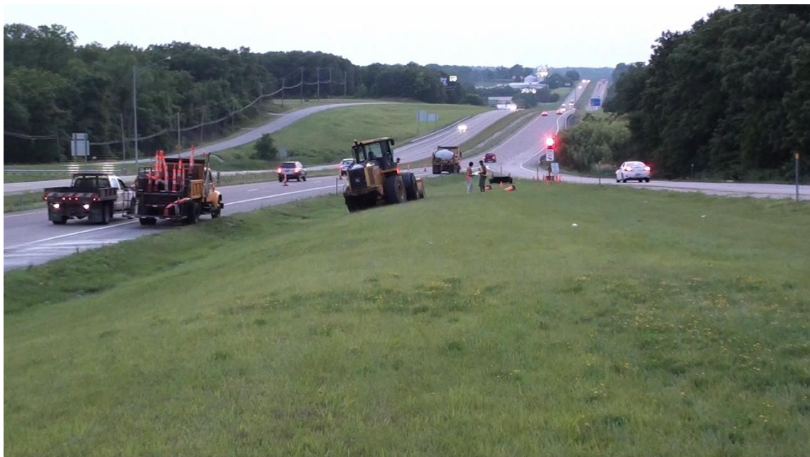
FIGURE 3.5 I-70WB @ mile marker 131, two-head signal.
