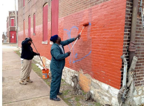
Illustration 39: City workers paint over graffiti on a building on the south side of the Forest Park Southeast neighborhood, March 2013.
