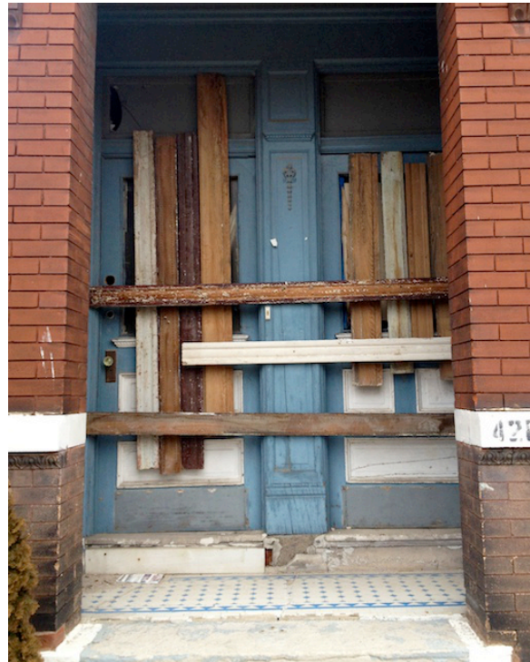
Illustration 11: A boarded door seals a home on Chouteau Avenue, September 2013.
