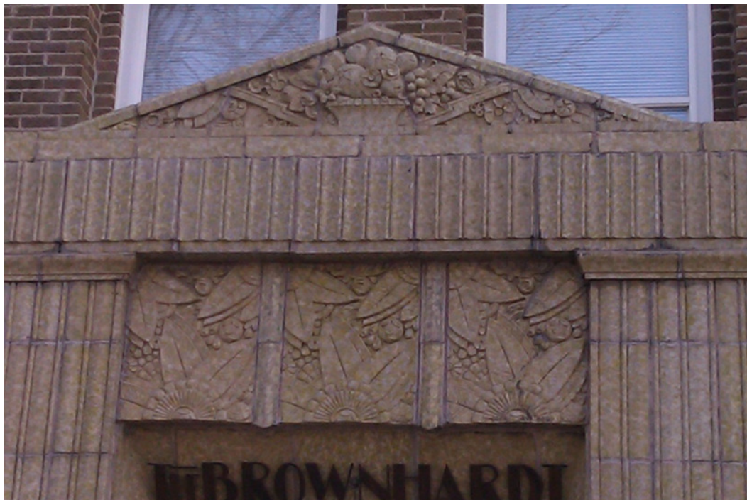
Figure 3.7. Detail of the terracotta overdoor featuring stylized lightning bolts and flowers in geometric patterns on the Brownhardt Apartments, 1929.
