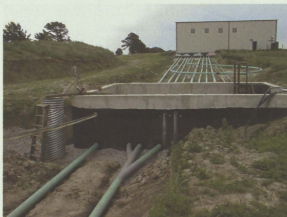
Coal log pipeline pilot plant under construction—This technology promises to revolutionize the coal transport industry. This is a project of Capsule Pipeline Research Center, University of Missouri-Columbia, U.S.A.
