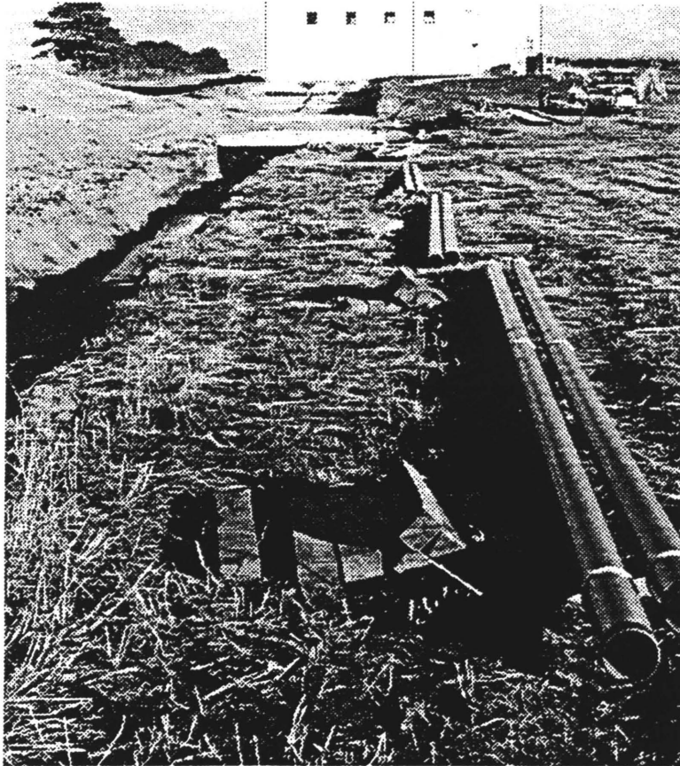
The pipes for the 3,000-foot 'loop' at the Holstein Farm wait to be placed. With such a large loop, researchers can recirculate coal logs indefinitely for testing.
