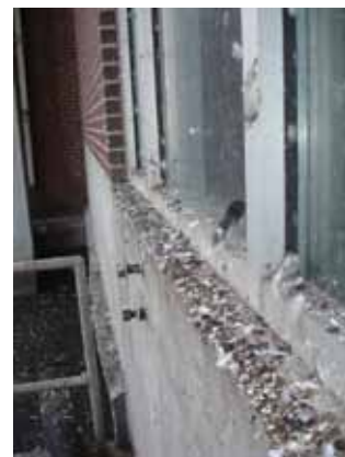
Figure 3. Pigeon droppings can be a health hazard.
