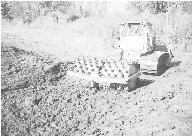
Figure 1. A sheep's foot roller provides the high degree of compaction often necessary to seal permeable soils at a pond site.
