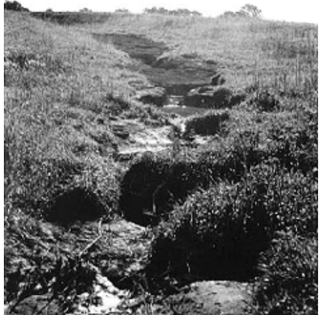
Figure 9. A livestock path can cause failure of the grass cover in the emergency spillway and, ultimately, if not repaired, dam failure.
