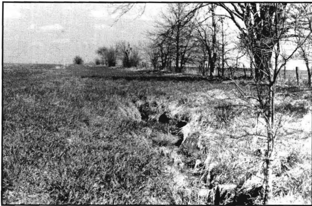
Brush and trees should not be allowed to compete with grass in the waterway. This unstable outlet may require regrading or a grade stabilization structure to eliminate erosion at the lower end of the waterway.
