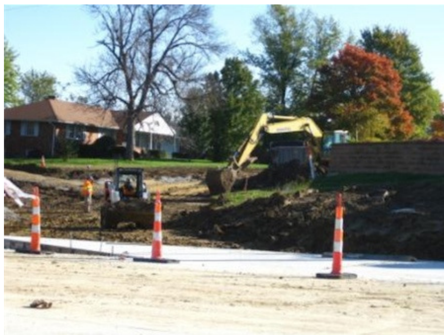
Figure 1: Construction at the intersection of Smiley and Rangeline in Columbia, MO. Photo by Marie Kersey
