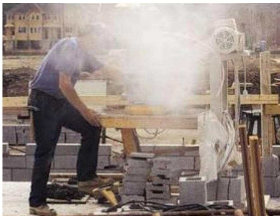
Figure 2: Fugitive dust blown into the air from a concrete saw. (Slate Health and Safety)
