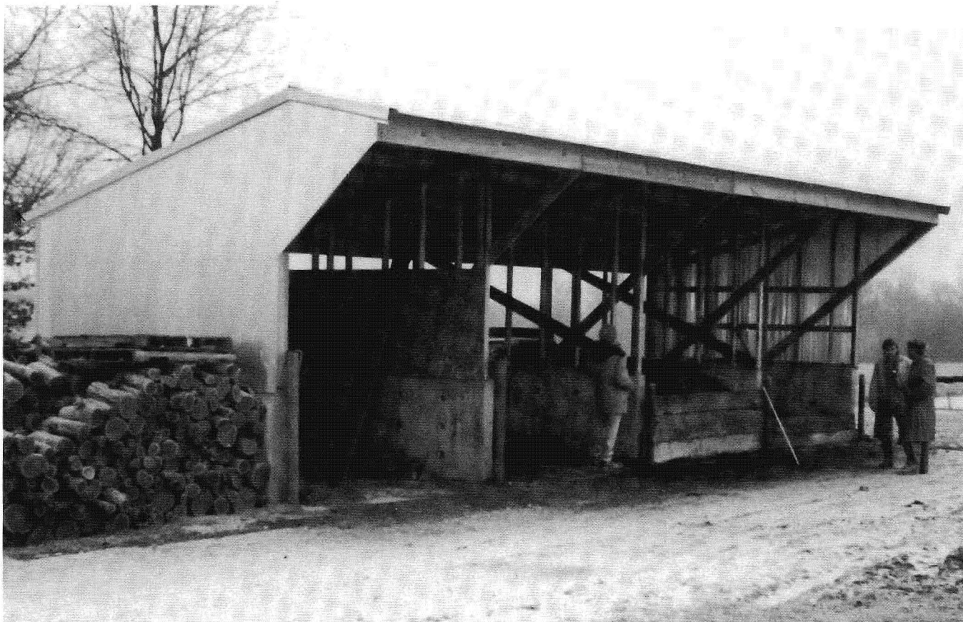
This roofed composter has concrete bin walls with a roof overhang to protect the work area.
