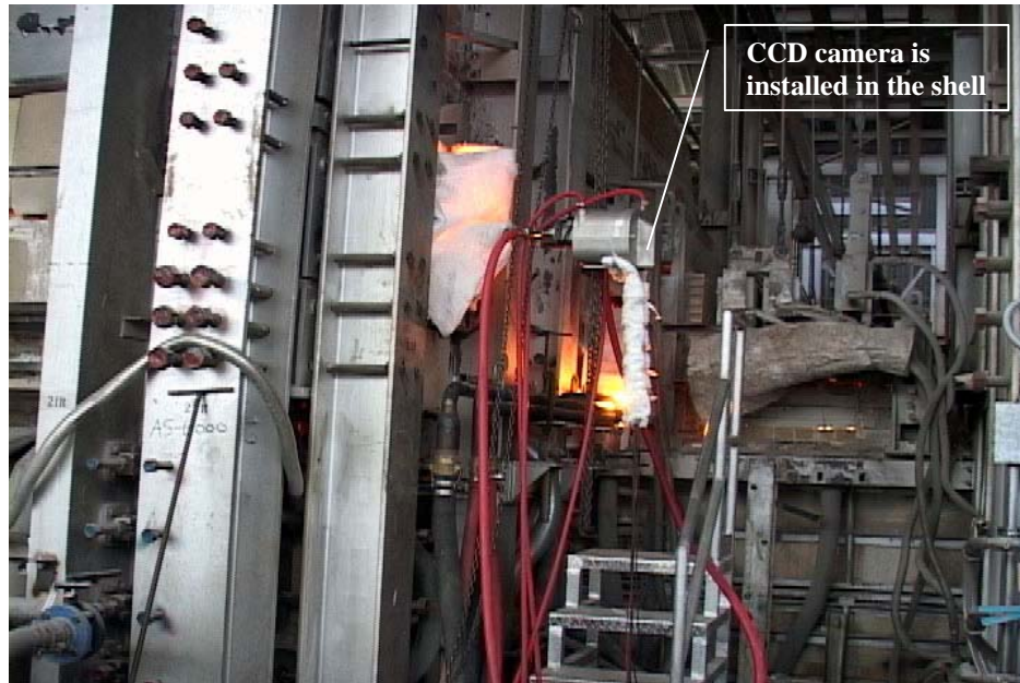
Figure 5.1 CCD Camera System Installed in Industrial Furnace
