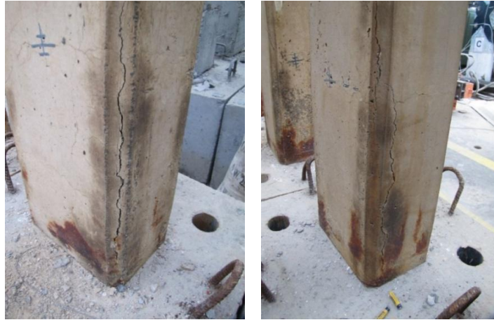
Figure 4.3: Photos of the cracked sections on specimens.
