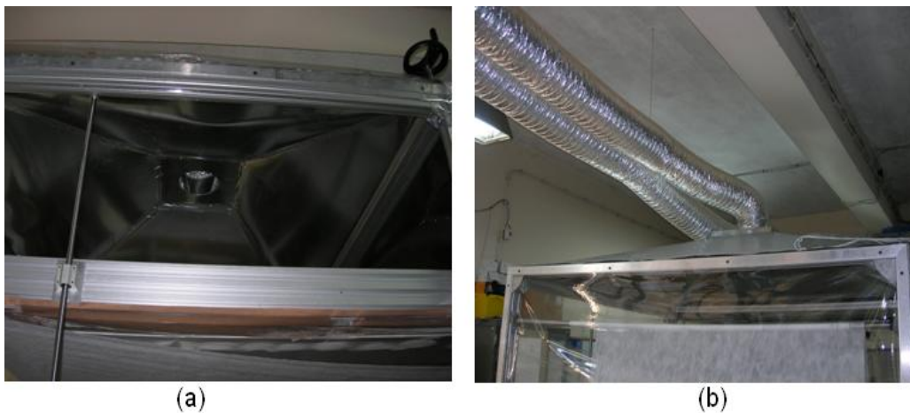
Figure 5.21 : a) exhaust hood b) flexible aluminum ducts.
