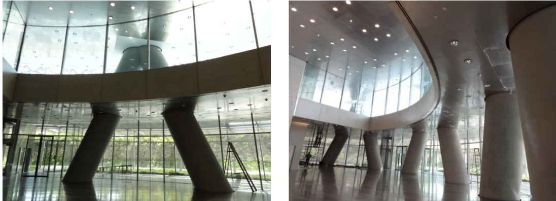
Figure 4.42 : Non-traditional concrete dia-grid with canted columns forming an X-shaped framing system (Author).
