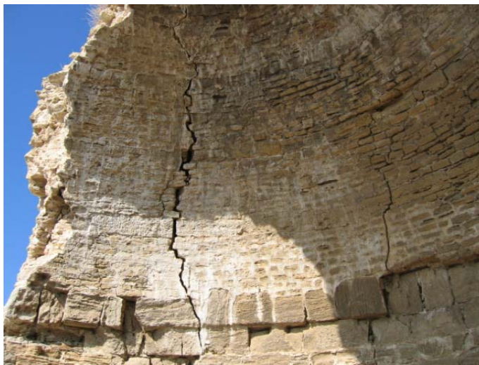
Figure 7.15 : Large crack (left) and capillary crack (right) observed on South Tower [10].
