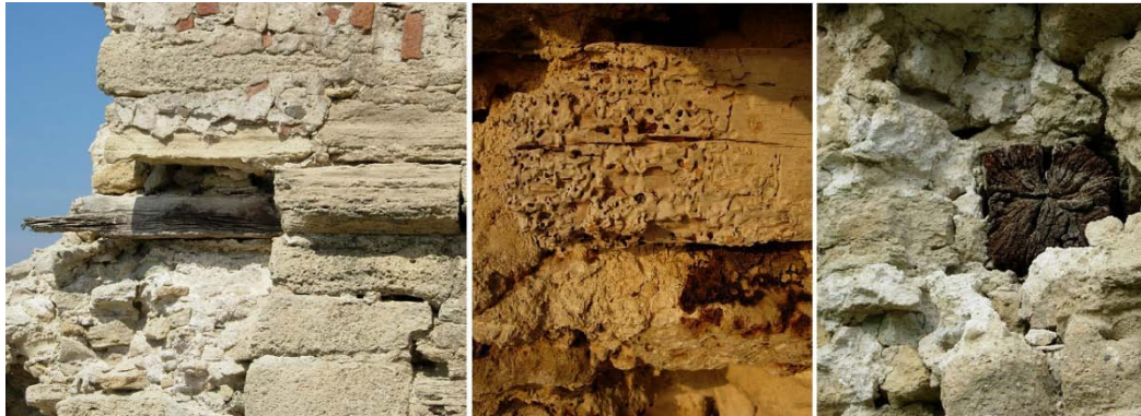
Figure 7.4 : Deteriorated wooden beams [10].
