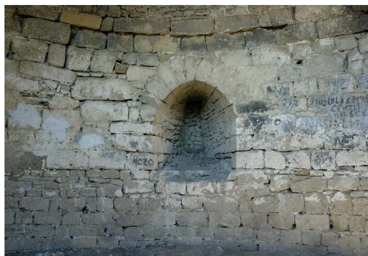
Figure 7.6 : Graffiti and paints observed on walls [10].
