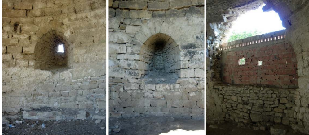
Figure 2.7 : East porthole (left), north porthole (middle), west porthole (right)[10].
