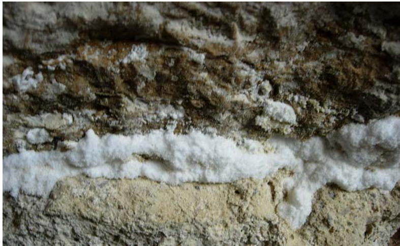
Figure 7.2 : Efflorescence observed on stone surface [10].
