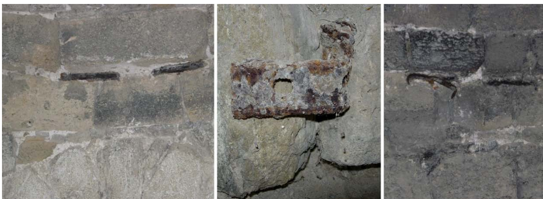
Figure 7.3 : Corroded metal clamps observed on façades [10].
