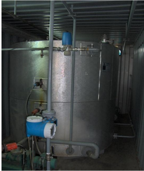
Figure 4.4: View of the anaerobic digester
