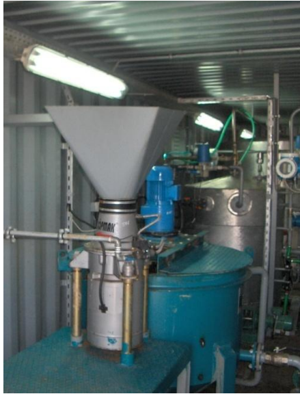
Figure 4.1: View of the Grinder
