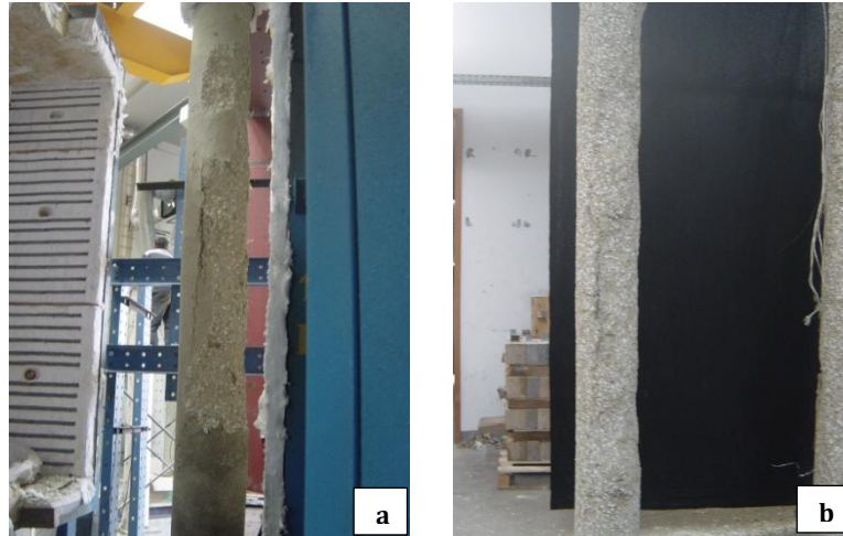
Fig.12 Concrete spalling after testing.
