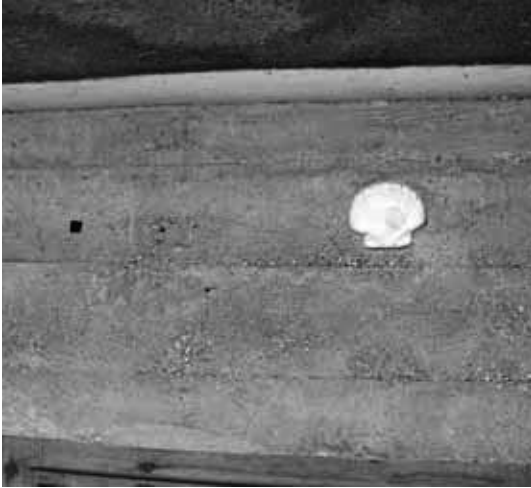
Figure 3. Detail of one of the concrete beams of the Ofir House. (Photograph by the author)
