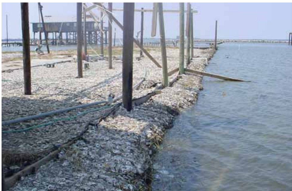
The Louisiana Sea Grant College Program deployed shell bags along eroded shore at its Sea Grant Oyster Hatchery in Grand Isle. Photo: Louisiana Sea Grant College Program/Louisiana State University
