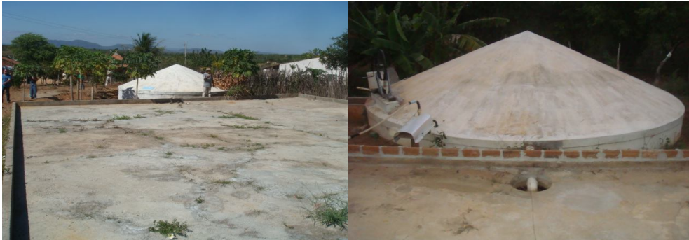
Figure 3 - Calçada cistern. The rainwater is collect on a constructed harvesting area and led to a cistern. Afogados da Ingazeira municipality, Pernambuco state, Brazil.
