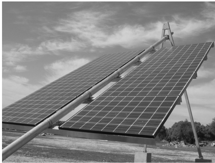
Fig. 4. Solar Park - motorized PV panels
