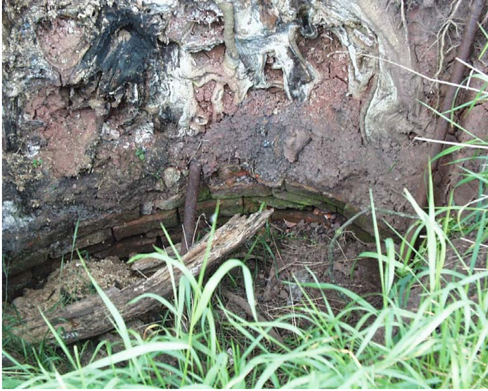
Fig. 10. Brick-lined mineshaft on Chilwell Dam Farm, (BNG 51285, 42342). Green algae on some brick suggests previously only partial light and possible recent collapse of the shaft cover.
