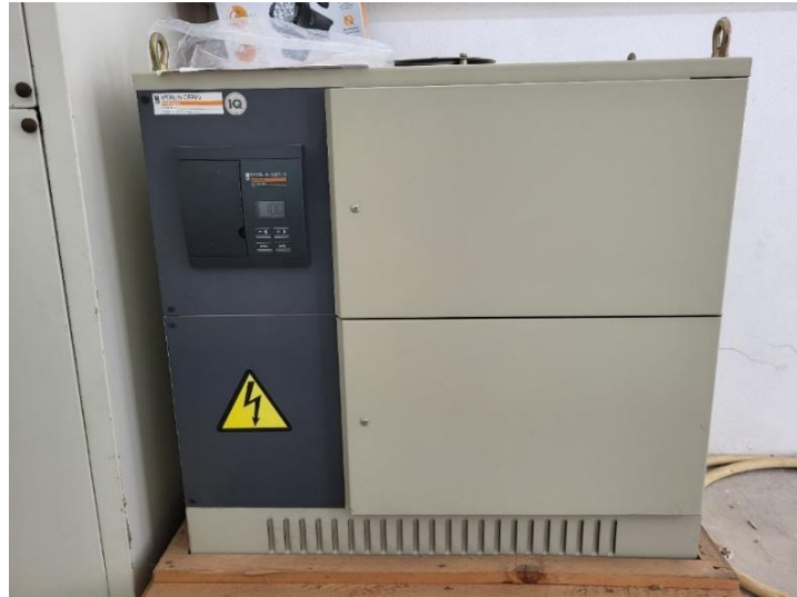
Figure 4.13 – Condenser bank PT1.
