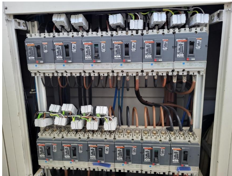
Figure 4.8 – Switch disconnectors and clamps.
