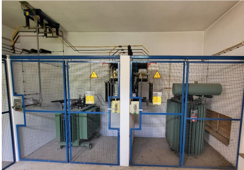
Figure 4.4 – Transformers A and B.
