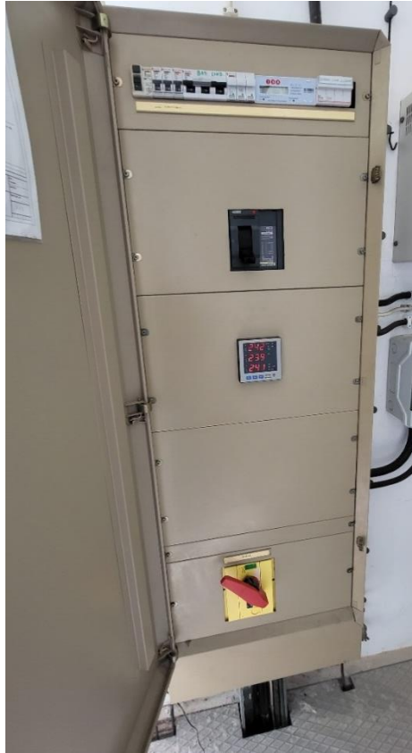
Figure 4.12 – PT2 electrical board.
