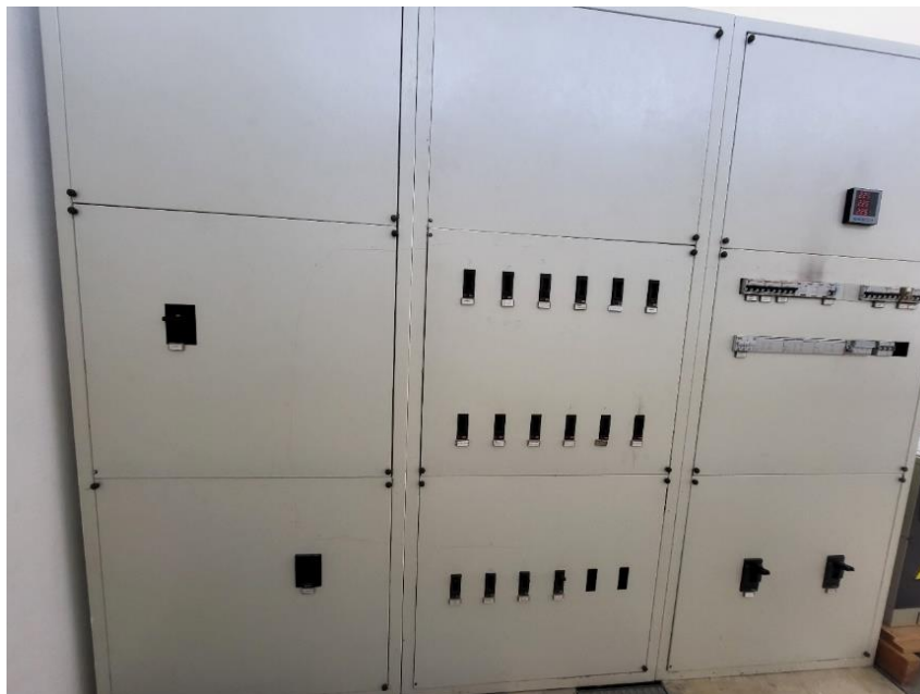
Figure 4.7 – PT1 electrical board.
