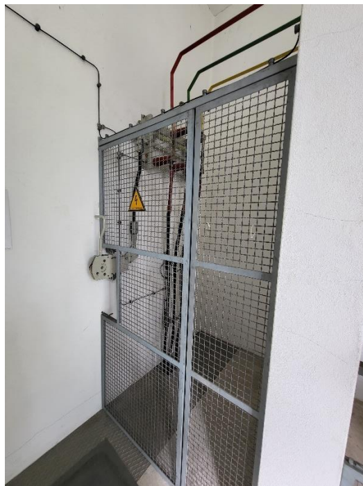
Figure 4.9 – 15kV cable emerging on PT2
