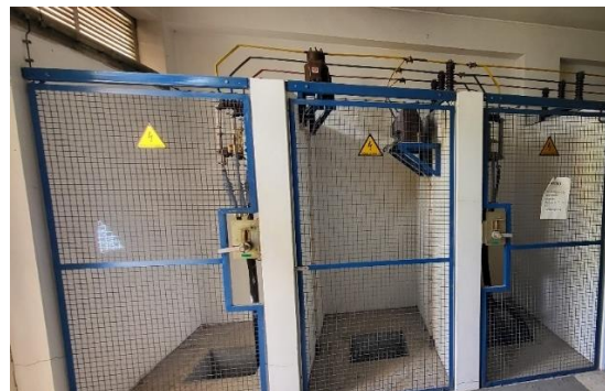
Figure 4.3 – 15kV cable in surface.
