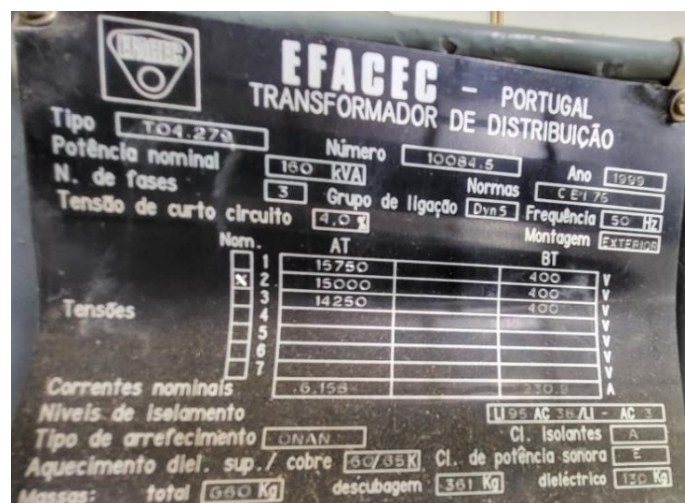
Figure 4.11 – Nameplate Transformer PT2.
