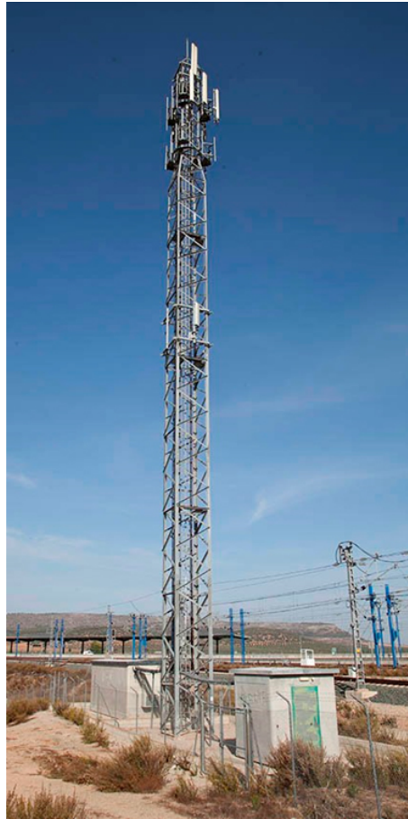
Figure 4.25: Tower structure with the eNodeB antennas installed at a height of 20 m. Two cabins are deployed, one for the GSM-R infrastructure and the other one for commercial telecommunication operators.
