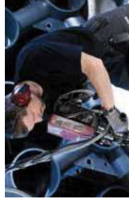
Extruder- and butt-welding PE is a proven and strong method of joining piping components.
