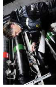
All installations are carried out by certified welders which ensure accurate and quality assured installations of PE 100 pipes.
