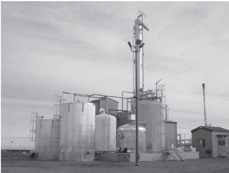
Figure 4. First commercial full-scale unit for biotechnological \text{H}_2\text{S} removal from high pressure natural gas. The Shell-Paques unit is designed to meet a \text{H}_2\text{S} specification of <4 ppm volume on the treated natural gas.
