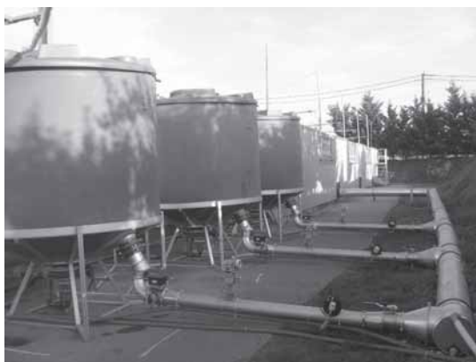
Figure 1. View of the three pilot plants and air pipes network.
