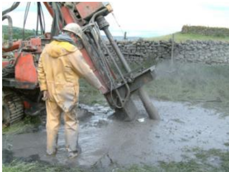
Figure 5 Five inclined boreholes to 50 m were drilled before spudding Eastgate with the aim of locating the Slitt Vein in the subsurface (photo by Paul Younger).
