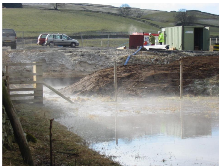
Figure 7 Eastgate produced hot saline water on test pumping in February 2005 (photo by Paul Younger).
