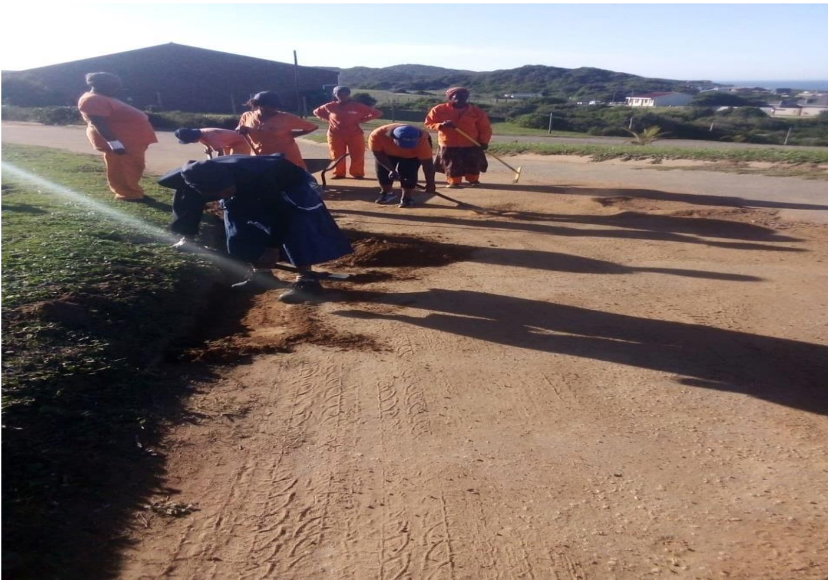
Figure 1.3: CWP general workers enclosing road potholes on road (Source: The picture was taken by the CWP Manager during one of the monthly site visits in April 2022)
