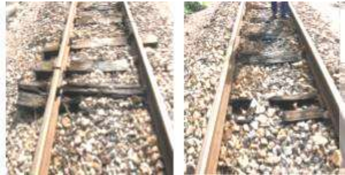
Figure 6: A dilapidated section of ZR.
