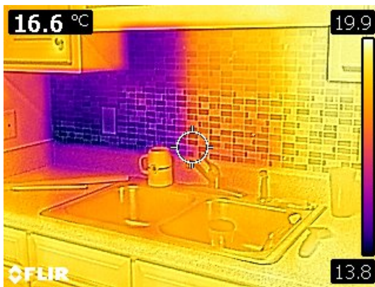
Figure 3: An exterior door with poor weather stripping (top), and an improperly insulated kitchen backsplash (bottom).
