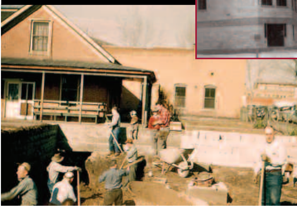
The Basque Center began with $40,000 in local donations and a ten-year high-yield bond. Pictured: digging the foundation, 1950. Inset: the cinder-block building as it appeared in the 1950s and '60s.
