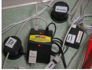
Fig. 3. Remote control relays used in activating power to thermal manikin sub-systems.
