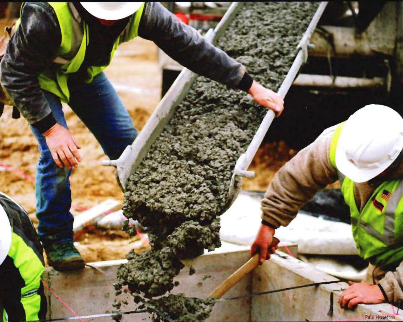
Economic development remains a goal of most cities, despite the slowdown caused by the Great Recession. Pictured: Boise construction workers. Next: Pueblo's Historic Arkansas Riverwalk.
