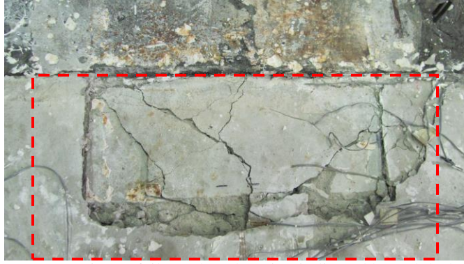
Figure 9: Approximate failure plane location indicated by red dashed line.
