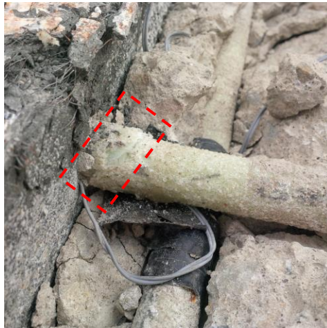
Figure 10: Shear failure of top GFRP bar after failure load adjacent to the closure strip.
