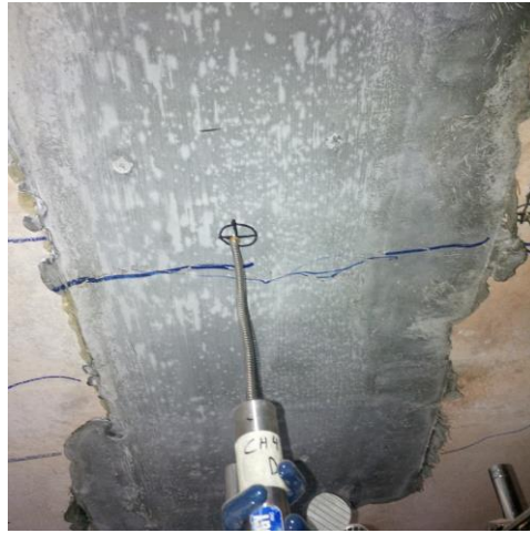
Figure 6: Crack through UHPC during fatigue loading adjacent to the closure strip
