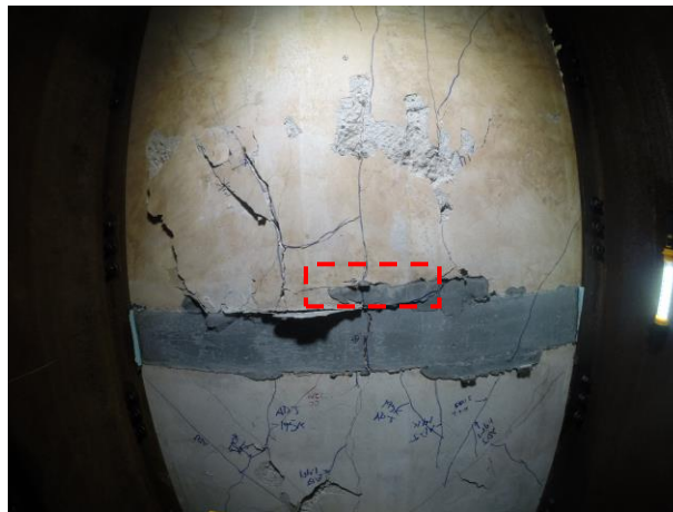
Figure 7: Underside of slab after loading to failure adjacent to panel (load location 2). Red rectangle indicates the approximate load location.
