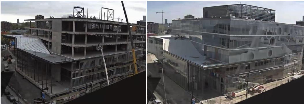
Figure 3: Construction sequence a) bare frame phase - September 2014, b) finished phase - July 2015 (Reproduced from (ÉTS 2015))
