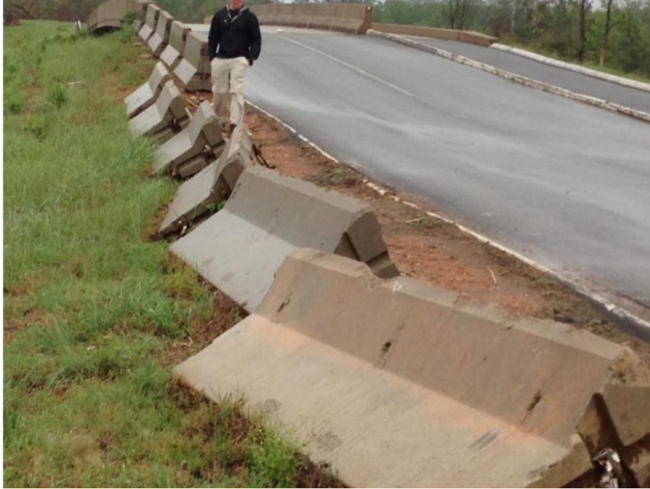
Figure 1: Overturned barriers from the Mayflower Tornado (Courtesy of Frank Lombardo)
