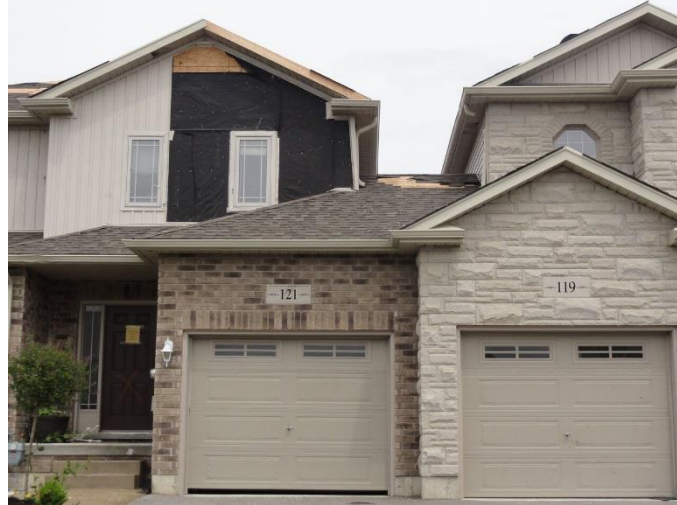
Figure 1: House from Angus, Ontario tornado with failure of vinyl siding.
