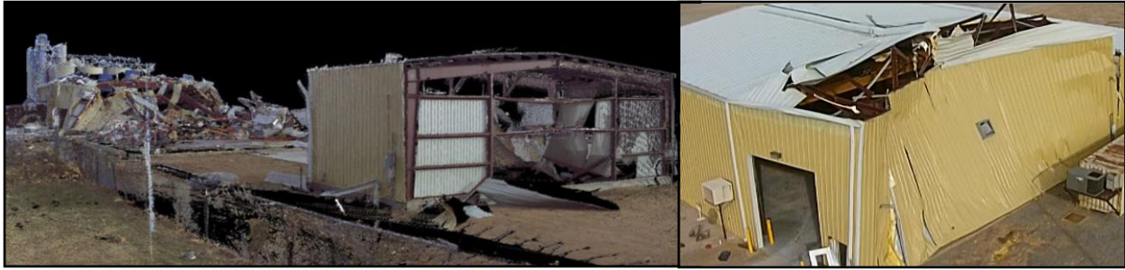
Fig. 6: LiDAR point-cloud data (left) and UAV imagery of damaged Halliburton facility at Pampa, TX (right).
