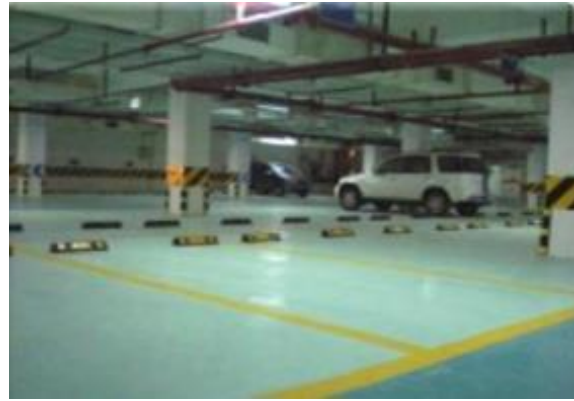
b) Self-leveling mortar cover with epoxy layer for floor covering of garage area
