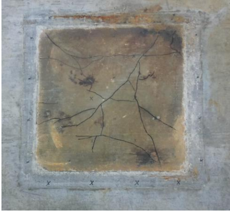
Figure 5: Corrosion-Cracked pattern on the corroded area
